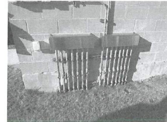
EAST EXTERIOR EQUIPMENT
